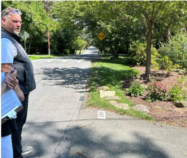
Problem: Water Floods the backyard via driveway.
