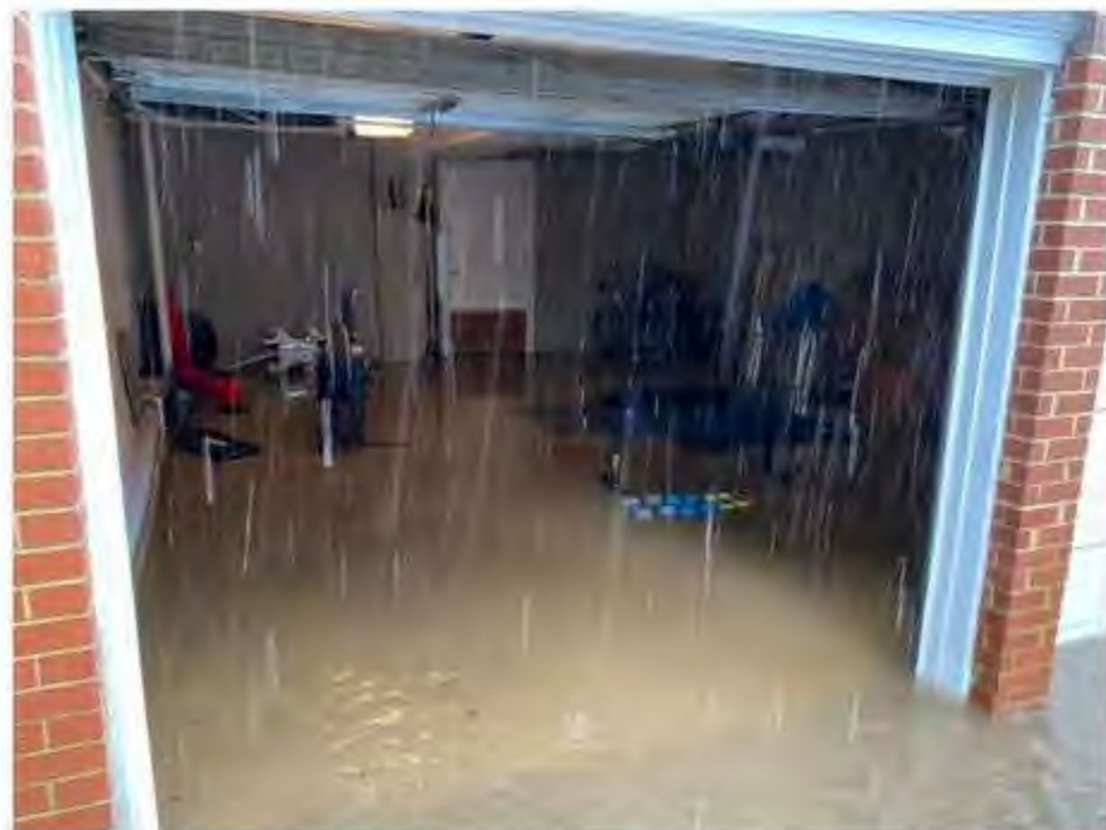
Flooded garage gym- water flowed from the street and down the driveway
